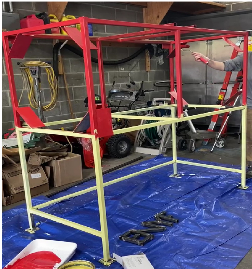
Paint to protect the metal
