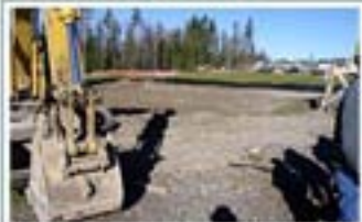
At Redmond Ridge, Quadrant Homes fences and protects existing forest as an amenity and stormwater filter. Then they grade to 12 inches below finish grade, stockpiling the topsoil. Next step is to place rock pads for roads and driveways.
