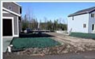
Once foundations are in and houses are framed and sided, 14 inches of compost-amended reused soil is placed (to allow for settling to 12-inch finish grade). The compost blend prevents erosion, so work can proceed year-round.
