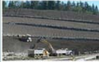
At Issaquah Highlands, Port Blakely Communities uses compost blankets for erosion control and cost-effective vegetation establishment on slopes.
